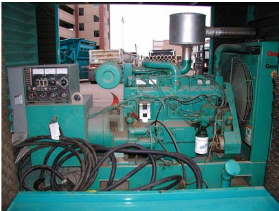
Photo ID: WW-05-2011Budget Capital Project: Trailer Mounted Generator
