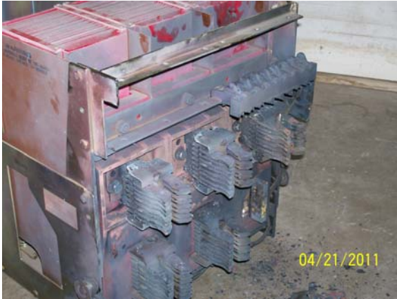
Photo ID: WW-04-2011Budget Capital Project: WRF Electrical Upgrade
